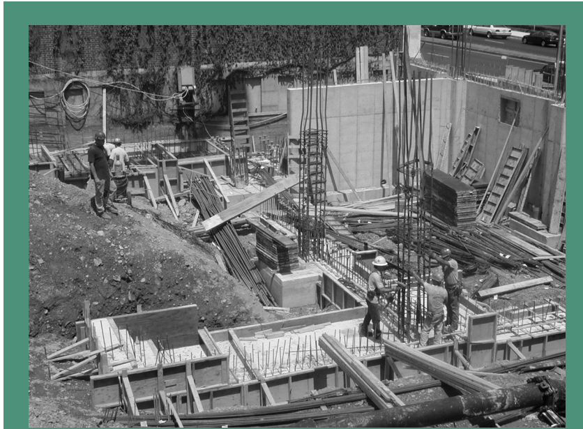
Work on the new building is moving ahead at a rapid pace. If you wish to follow progress, consult the "Construction Project Update" section of the Society's website: www.americanantiquarian.org . Be a part of the project by making your gift to help AAS claim the Kresge Foundation Challenge Grant.
